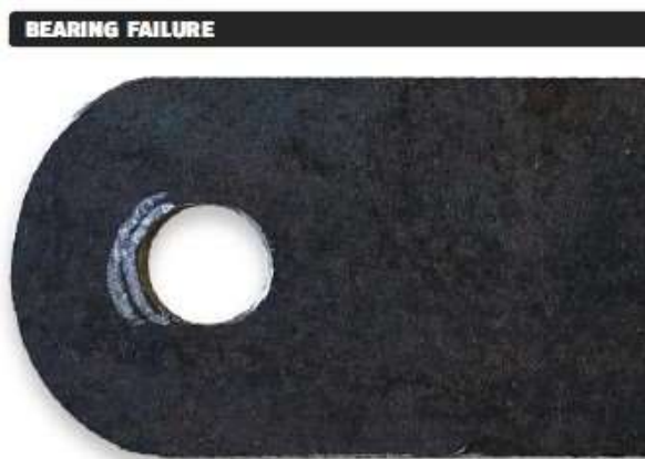
A bearing failure occurs when the material is too thin for the size of the bolt and the load. It first presents as an oval hole.
